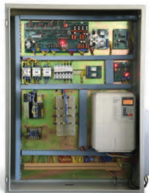
9SSVF Control System
